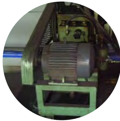
Hydro Testing M/C
